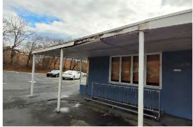
Deteriorating Fascia on the East Elevation
